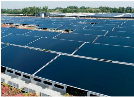
Fig. 10.a. Tectum flat roof PV system
