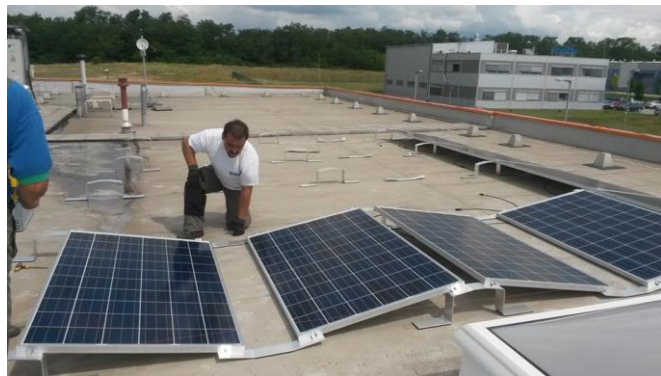
Fig. 10.b. Flat fixation of PV module installation, NVS (2014)
