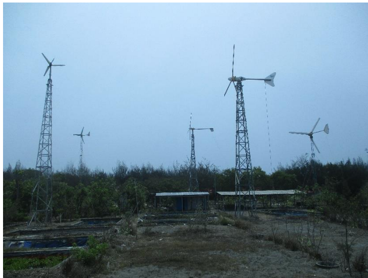
Fig. 7: Pantai Baru hybrid system of Wind-PV-Diesel for ice making (Source: Soeripno)
